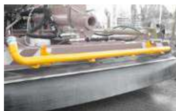
High pressure watering line, 4 sprayers
